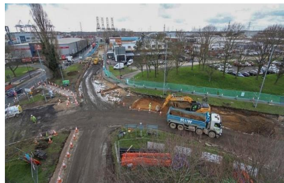
A major programme of road resurfacing and traffic signal upgrades including A33-A35 Millbrook Roundabout.
